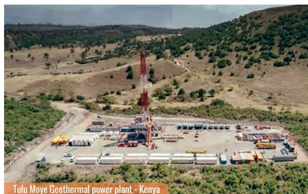
Tulu Moye Geothermal power plant - Kenya
